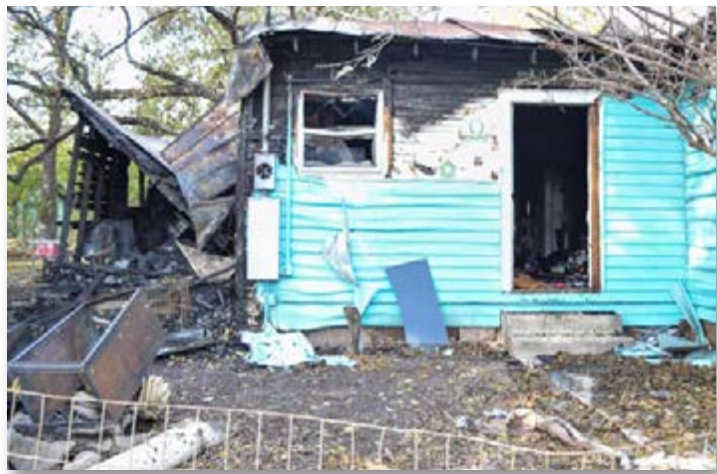
ALEXANDRIA RANDOLPH | DISPATCH RECORD This residence on East Fifth Street was deemed a "total loss" after a fire started in an exterior wall and burned the house on Tuesday morning. The two residents and their dog were unharmed.
