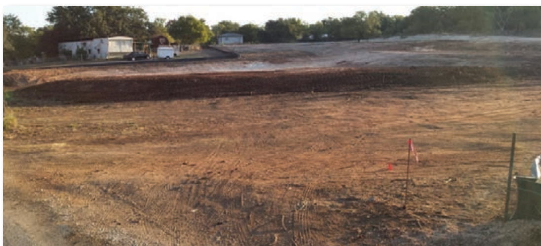
Land has been cleared for houses and a rainwater detention pond in what will be the Brodie Estates subdivision east of Brown Street, south of Cloud Street and northeast of Hillcrest Drive. Chris Harrison, one of the Brodie Estate developers, said all the infrastructure may be installed by the end of this year. The houses will be about 1,400-1,600 square feet, Harrison said.
