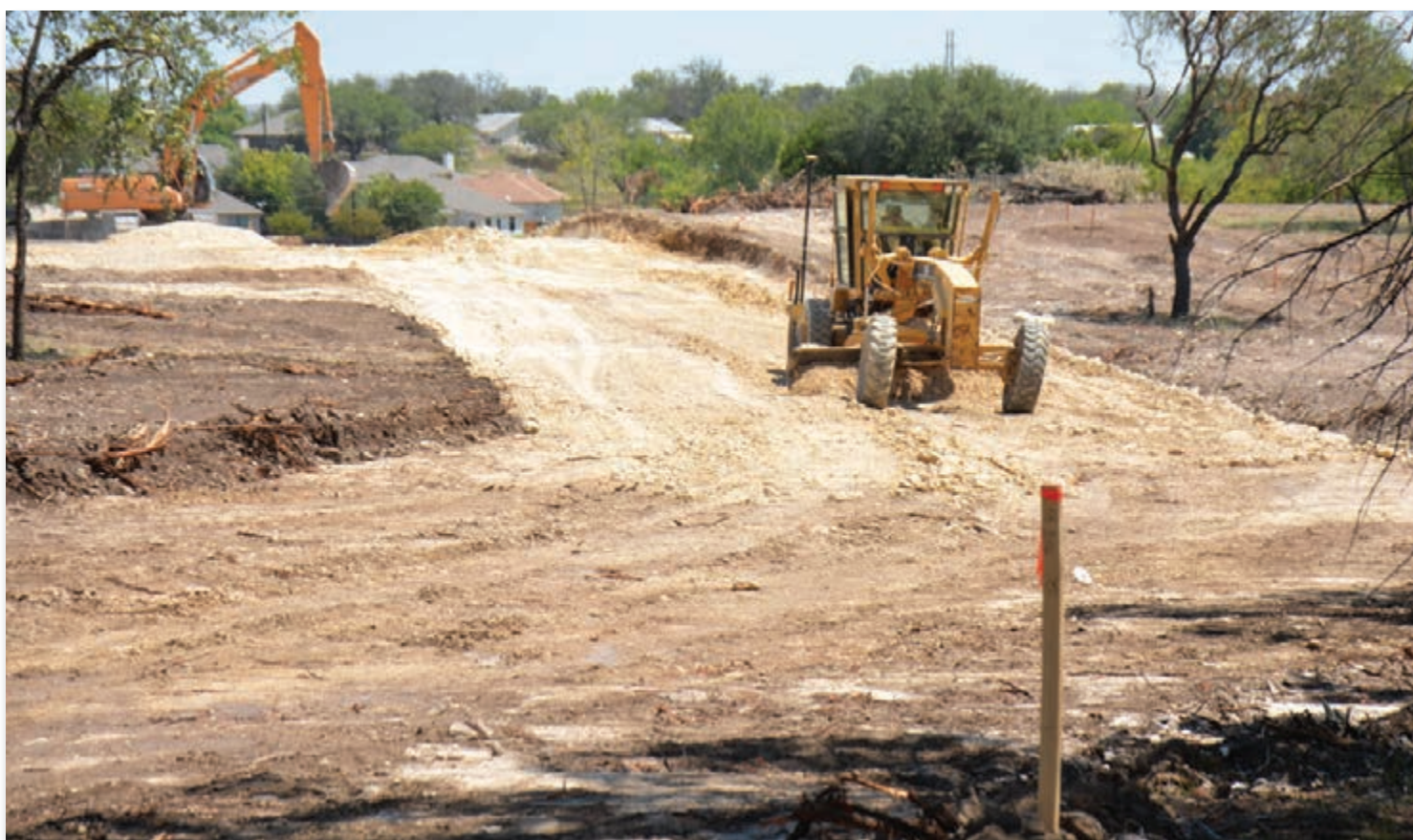
Road work began in August on property between Nix Road and North Willis Street, where developer Deorald Finney is constructing Stone Valley subdivision. Finney said he plans to develop in Stone Valley phases and ultimately put 67 single-family houses in the subdivision.
